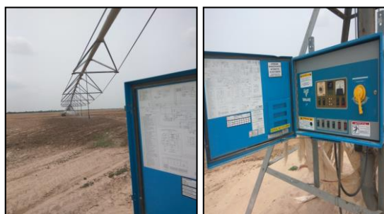
Fig 1: Control Panel of Center pivot irrigation system equipped with a backflow prevention valve used to apply irrigation water, at Central State Farm, NSC, Ltd., Sardargarh, Sriganga nagar, Rajasthan India
