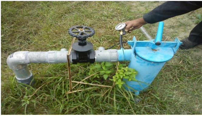
Fig 3.3: Screen filter and pressure gauge
